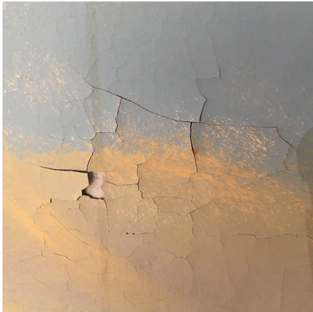
Detail of Lifting and Flaking Paint
